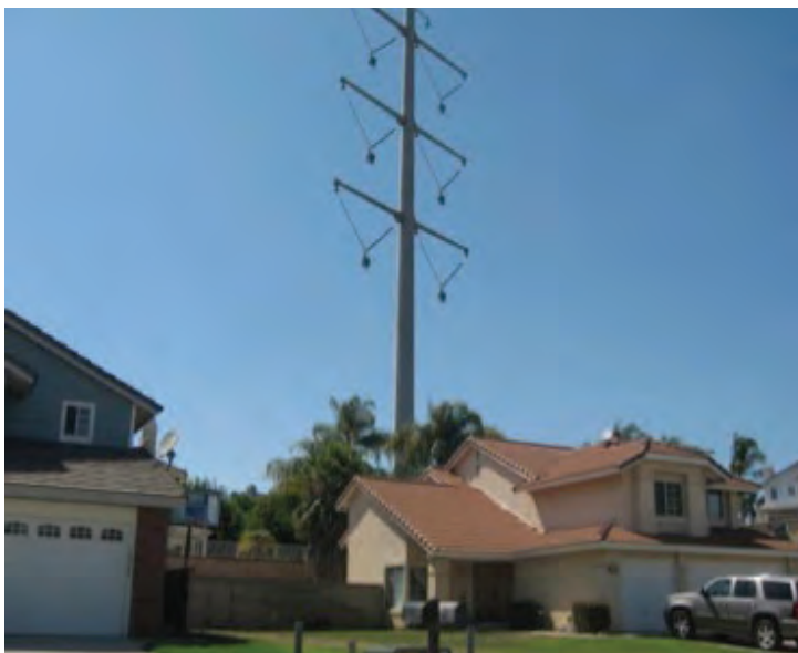
Residents in Chino Hills persuaded the Public Utilities Commission to suspend construction and underground a 3.5 mile segment, causing $220 million in incremental legal and construction costs.
