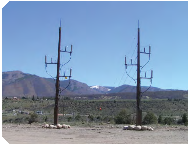
These towers bring the 115 kv line across the Roaring Fork River where it goes immediately under ground to begin its seven-mile journey under Highway 82 to the GIS substation.
