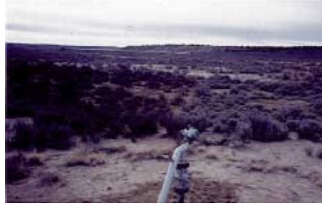
Photo A-2: "Dog leg" on a water well that blew and kept leaking. Note the oil soaked sagebrush.
