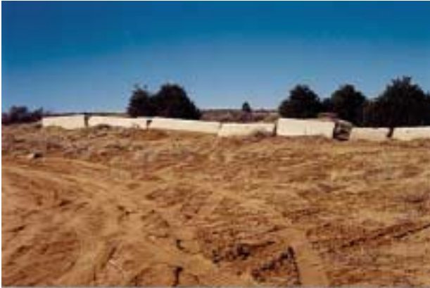
Photo A-9: Unremoved concrete blocks, discarded after use.
